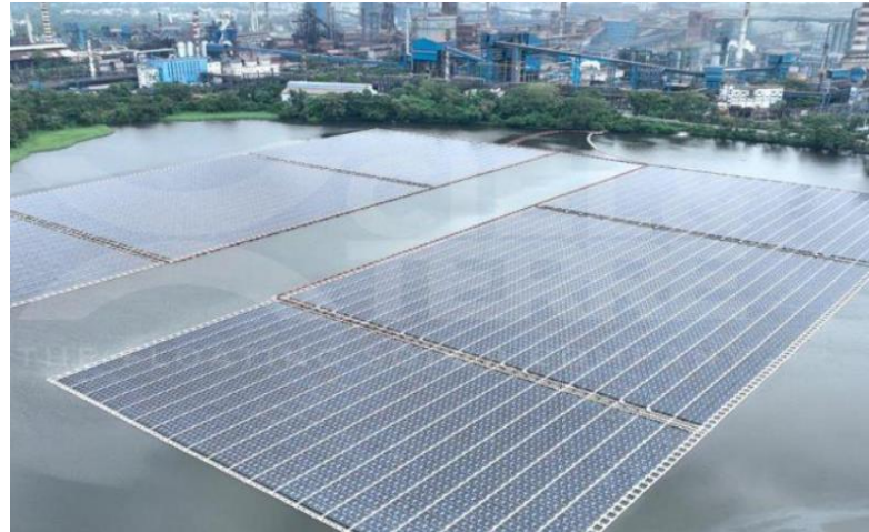
Floating Solar (10.8 MWp) commissioned at TSJ works in Sept'23.
