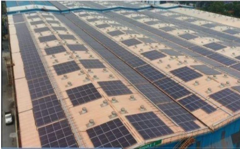
Roof Top Solar commissioned at TSJ.
